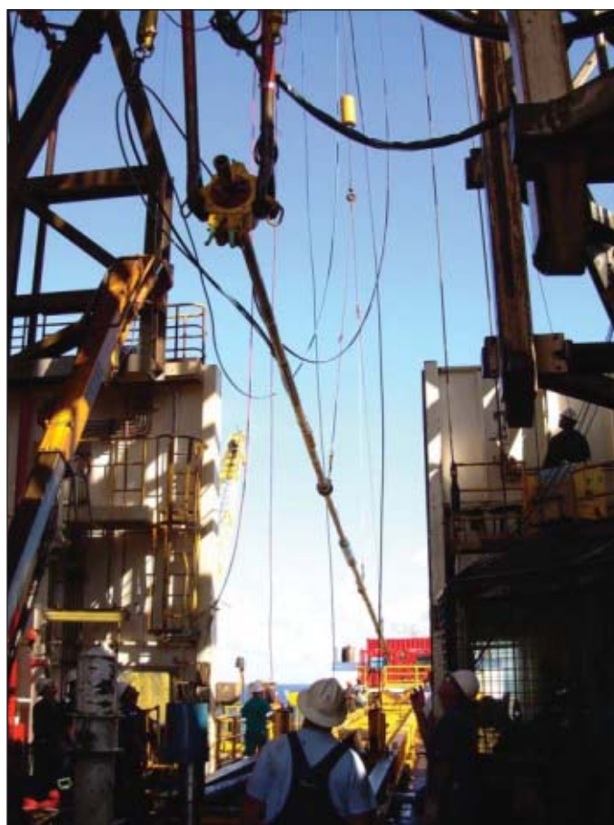
Rehearsing the process several times onshore proved valuable when lifting the BHA at the rig site (Fig. 4).
